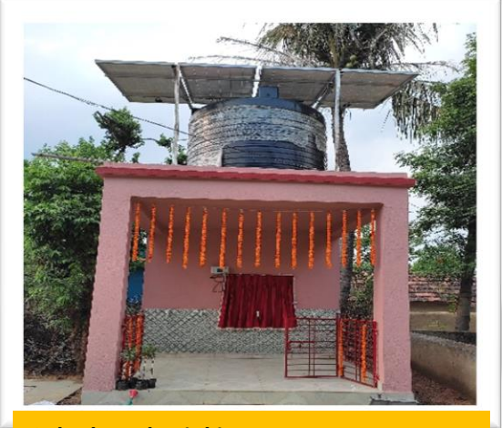
Solar based Drinking water system at tribal village Babuisole
