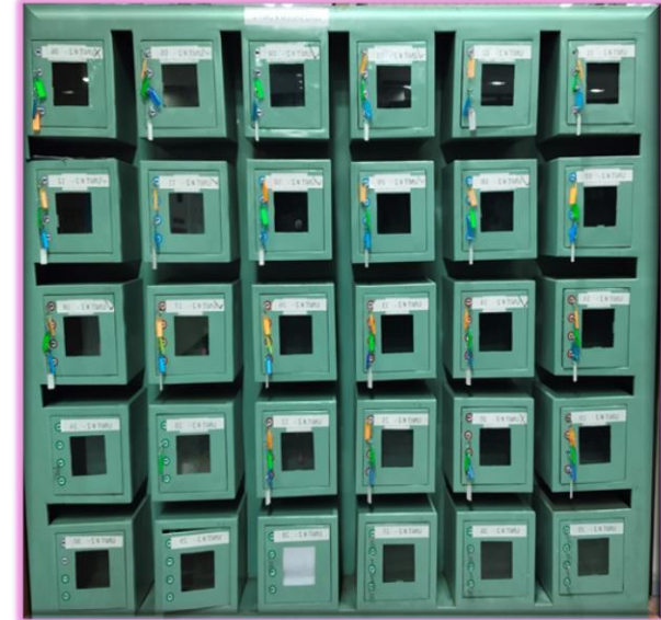
LOTO System for HT Breakers.
