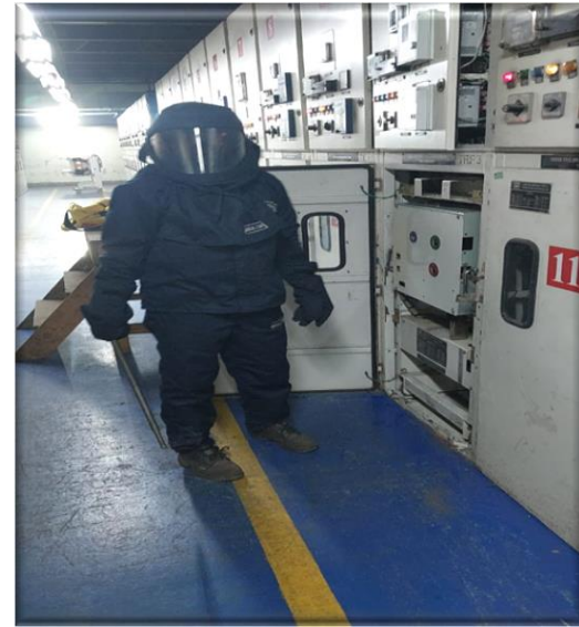
Arc Flash Suit for handling of HT Breakers.
